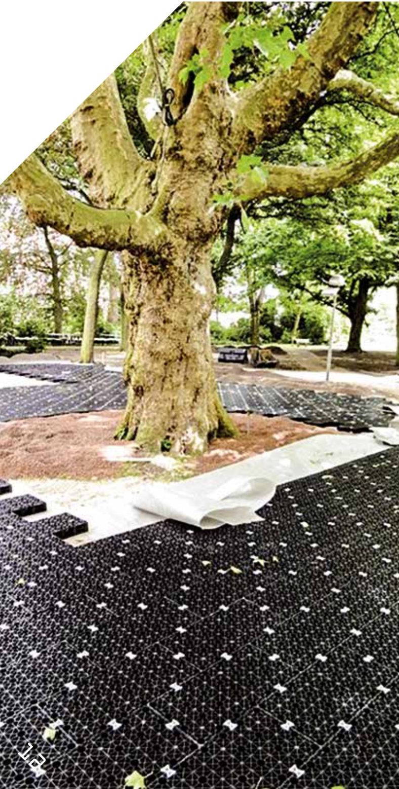
< Tolhuistuin Amsterdam. The Permavoid subbase is used under a semi-paved surface to protect the roots of a monumental London Plane tree when transforming a former garden into an event area.
